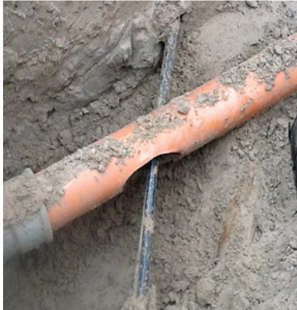
Figure 2.2: Damage to a lateral connection by a cross drill (Langeveld and De Haan, 2014).
