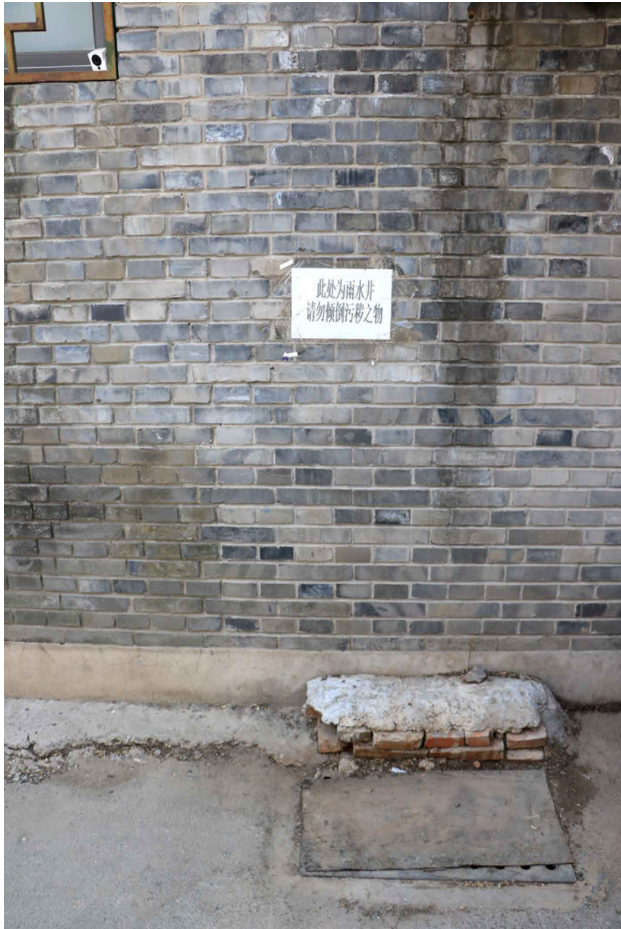
FIG. 6.4 The covered catch basin and the warning sign on the wall (source: author photo, 2019)
