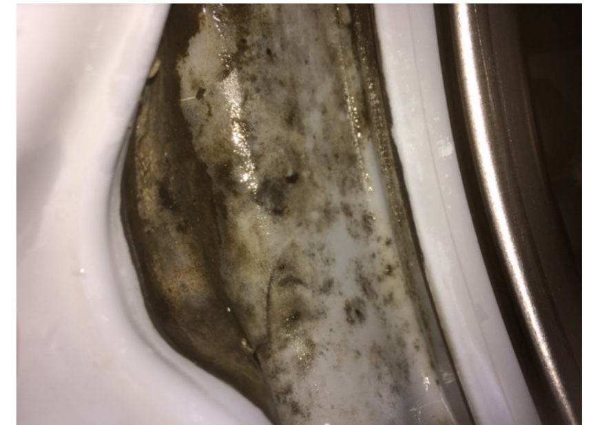
Image 11. Deteriorated and stained rubber ring
