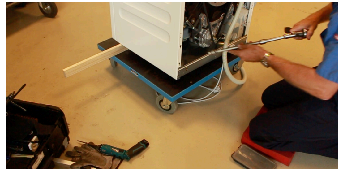
Image 16. Tool extension needed to reach the component.
