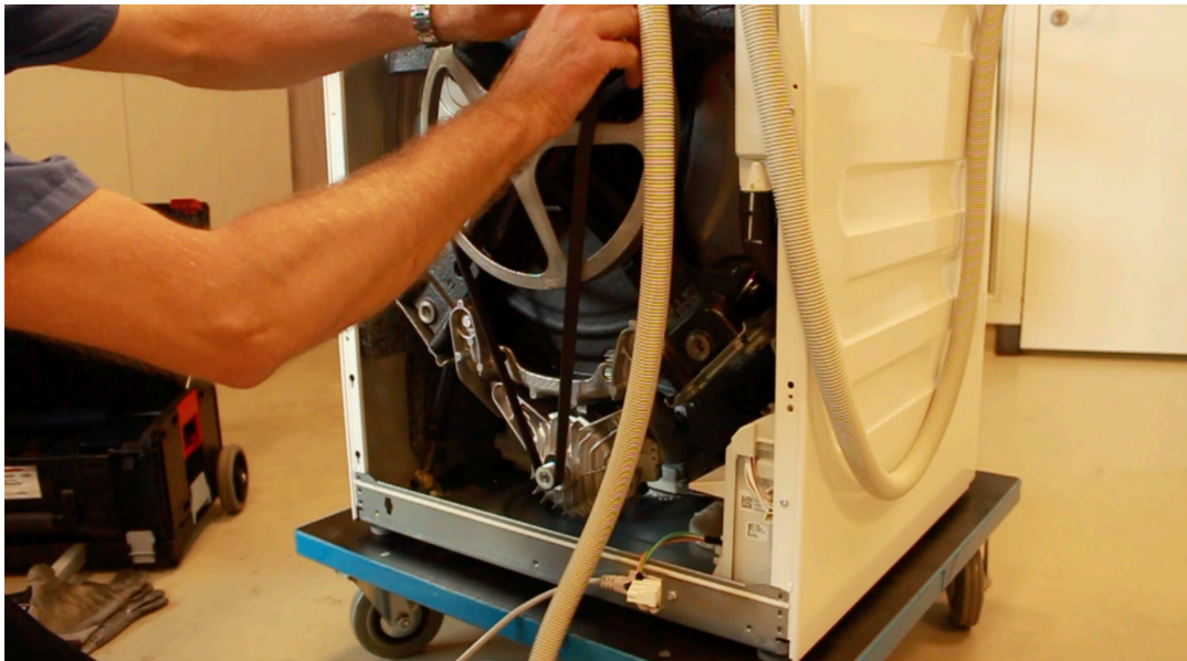
Image 19. Good visibility and good mobility for the assembly and disassembly of the belt.
