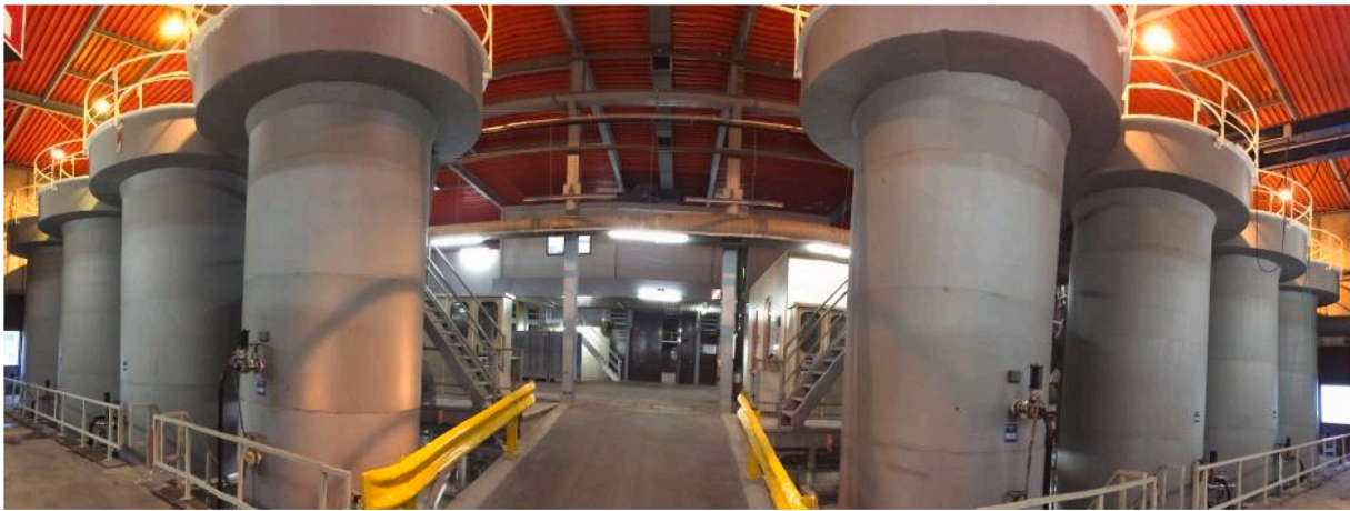
Fig. 1. Full-scale pellet softening reactors located at Waternet (Amsterdam, The Netherlands) [10].
