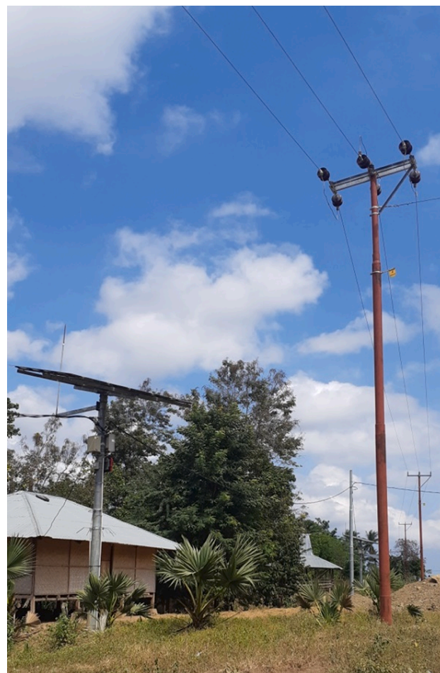
Fig. 3. The (almost) overlap of two electricity systems in rural Sumba Island – the PLN's grid (right) and the private off-grid solar system (left) (First author).
