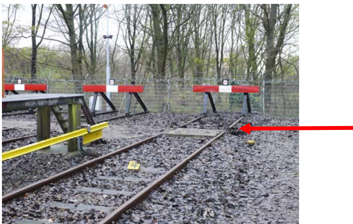
Figure 38. The damaged buffer stop at Gaasperplas terminus; notice the gap in the track
