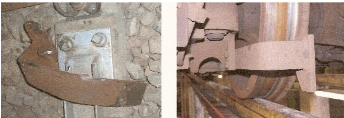
Figure 35. The dropped right-hand catcher as found (left) and as normally mounted (right)
