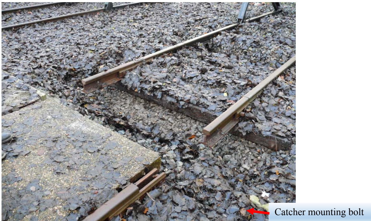
Figure 40. The gap in the track caused by the collision with the buffer stop
