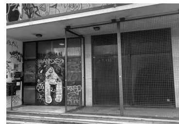
Unwelcoming and derelict entrance
