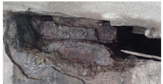
Figure 3 Corrosion of the steel support.
