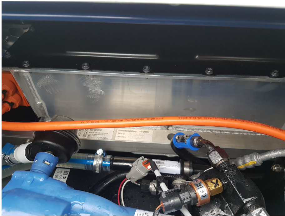
Figure 4.4: Lithium battery system.
