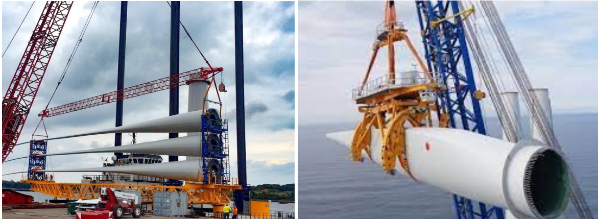
Figure 3.6: A blade rack that can hold 3 wind turbine blades. Figure 3.7: A wind turbine blade lifted with a blade yoke.
