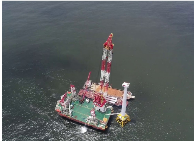
Figure 2.10: Installation of 5.5MW turbine for the Yangjiang Nanpeng Island Offshore Wind Farm
