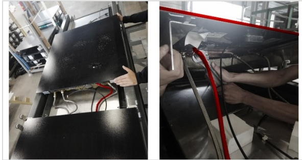
Figure 99: Fixing of the cooper pipes (right) and the placement of them one after the other (left).
