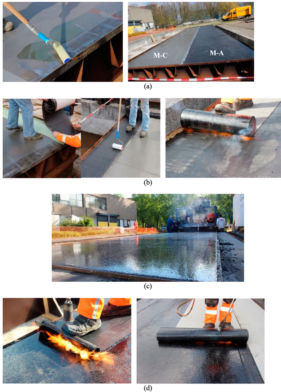
Figure 4. Construction steps of the superstructure; (a) application of Primer at the top surface of steel deck on both membrane sides (i.e. A (M-A) and C (M-C)), (b) first membrane layer on M-C (left) and M-A sides (right), (c) GA at the top of membrane layer, (d) second membrane layer on M-C (left) and M-A sides (right).
