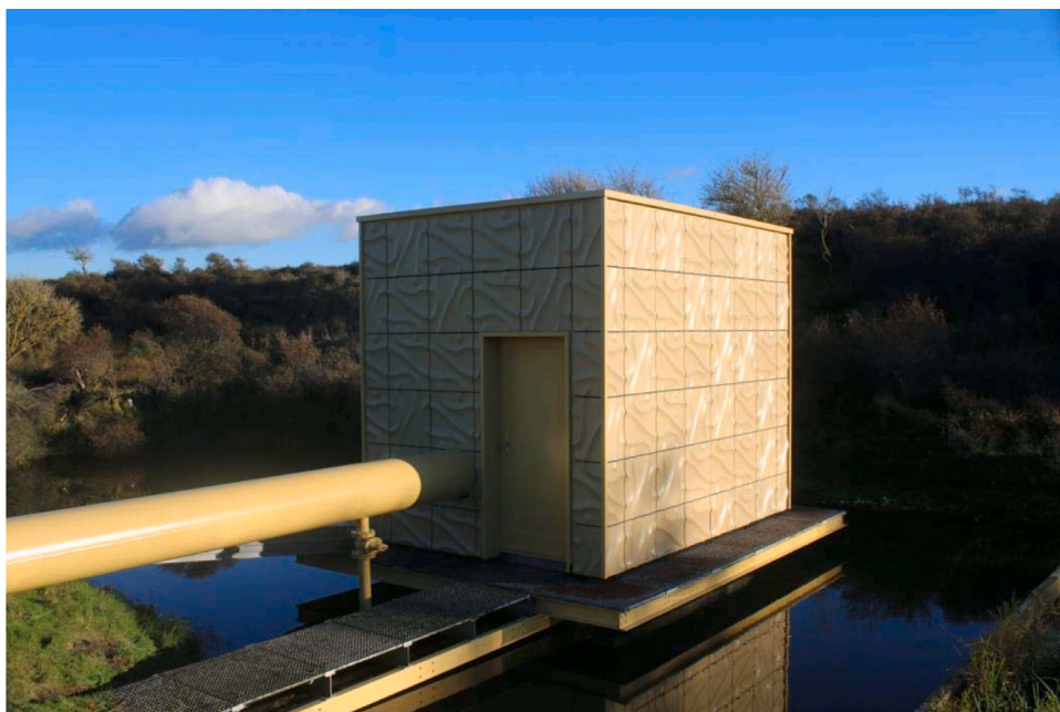
Fig. 3. Façade panels applied at the pumping station in a natural reserve [picture from D1.9 WIDER UPTAKE report].
