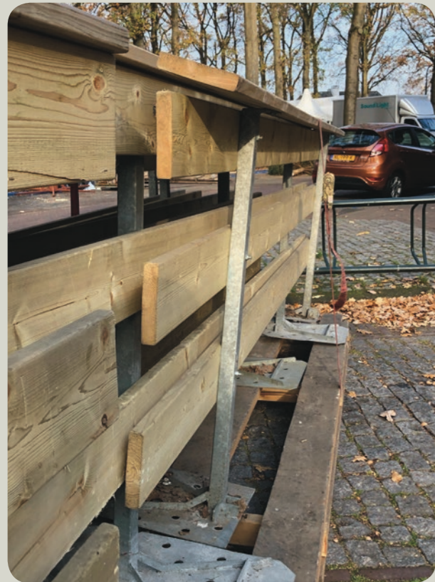
Image 23: Clamping straps deform the boarding construction. Source: Author.
