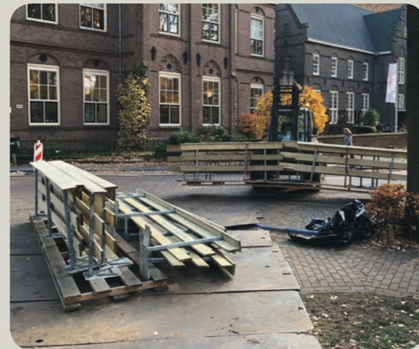
Image 24: Instable boarding and moving a pallet with boarding. Source: Author
