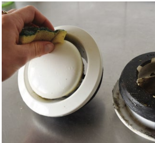
Figure 11 Residents are expected to clean the valves. But cleaning them without adjusting configuration or mixing up valves is a challenge
