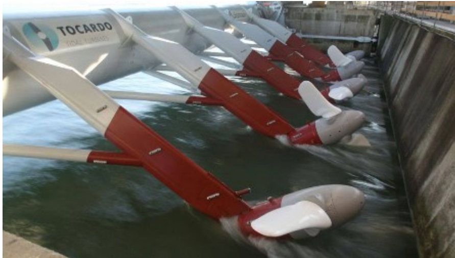
Figure 1.3: Tocardo's installed HATT's in the Eastern Scheldt storm surge barrier from [3]
