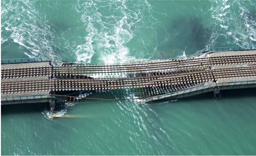
Figure 1. Malahide Bridge Collapse (21 st of August 2009)
