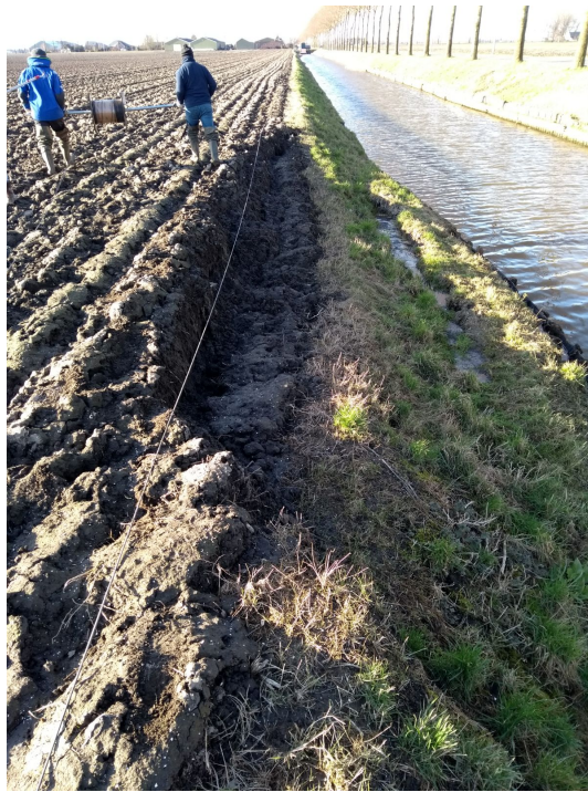
Figure 2.12: A collapsed bank caused by one of the boils which is detected in the Lissertocht
