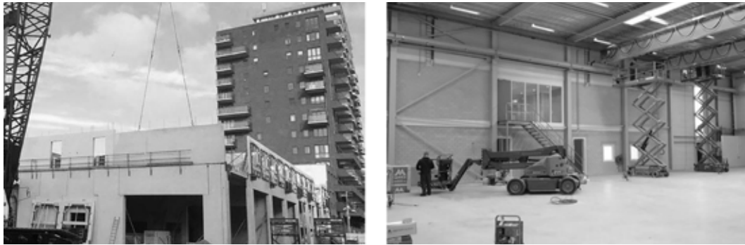
FIGURE 11 Under-construction housing tower building project of case B (left), and the interior of utility building of case C (right).
