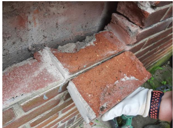
Figure 124: Location 2 Brick 2 Collapse Method
