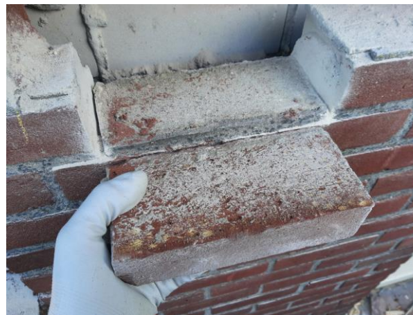
Figure 115: Location 1 Brick 1 Collapse Method
