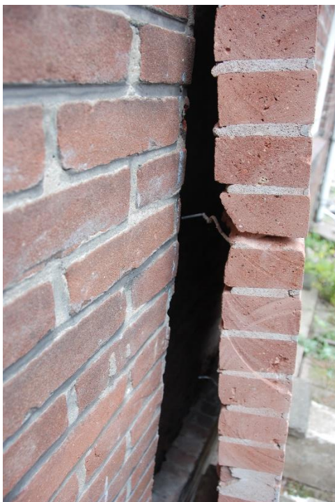
Figure 148: Wall ties still is connected to the outer leaf
