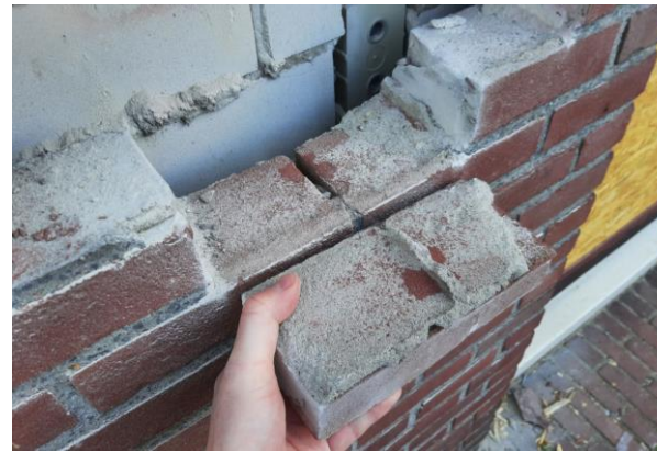
Figure 119: Location 1 Brick 3 Collapse Method
