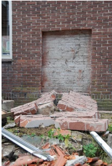
Figure 152: Ruins of element location 2
