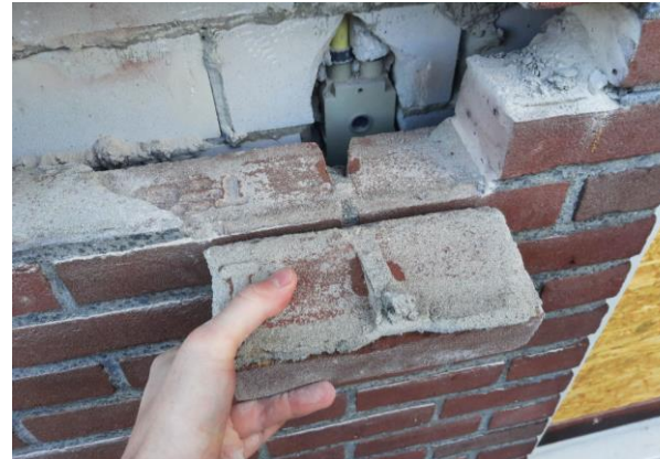
Figure 117: Location 1 Brick 2 Collapse Method
