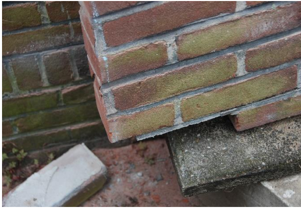
Figure 146: Damage to bottom left brick
