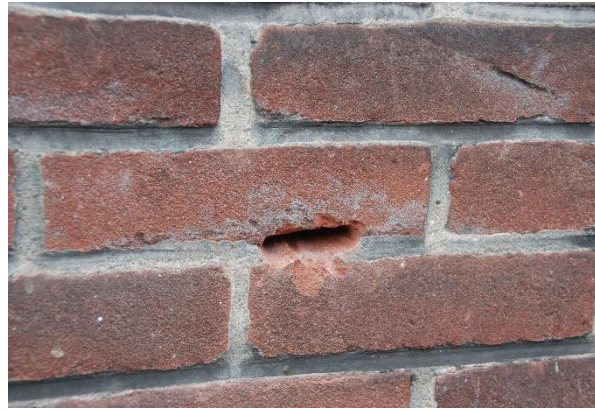
Figure 147: Damage due to removal of wall ties
