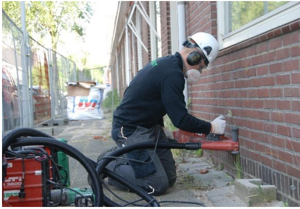
Figure 127: Location 1, ower saw cut
