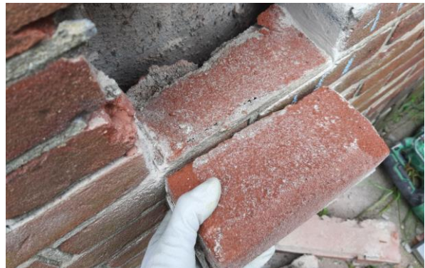
Figure 122: Location 3 Brick 1 Collapse Method
