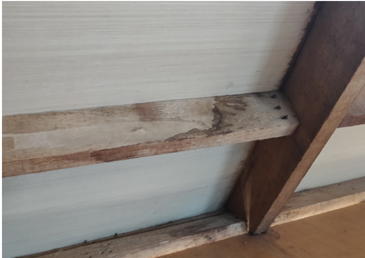
Figure 11: Moisture in rafters and battens due to water from the roof opening
