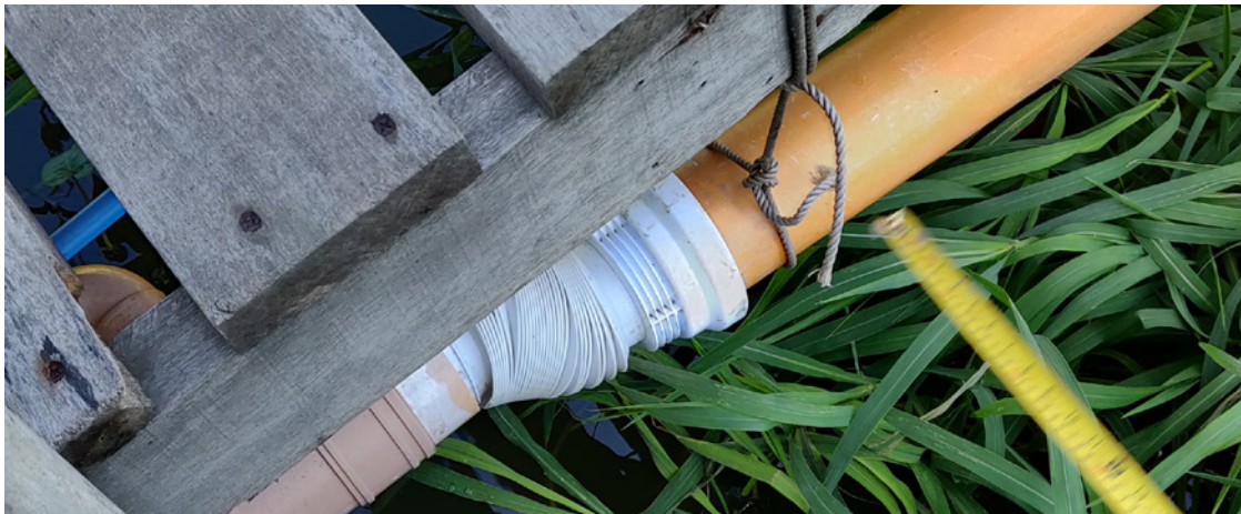
Figure 09: Leakage in the pipe to septic tank
