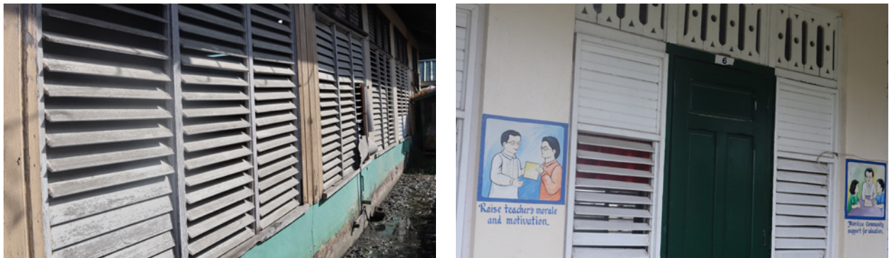
Figure 24: Louvers used for the opening in a school building built in 1940s, Macabebe
