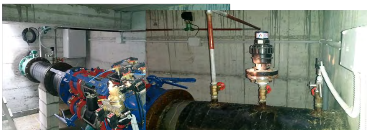
c. PRV chamber, from inside
