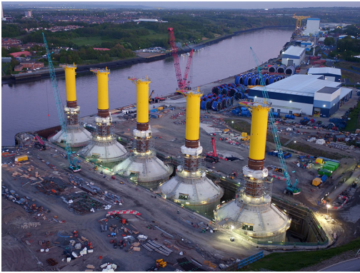
(a) Aerial view of the construction site at the Port of Blyth. The five GBF's were constructed simultaneously in a dry-dock. Image is from: ( www.bam150years.com , n.d.).
