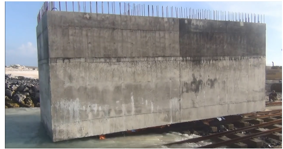
Figure 1.13: A caisson is lowered into the water on an inclined slipway equipped with rails. The motion is restricted by cables and winches. Image is from: (YouTube, 2017).
