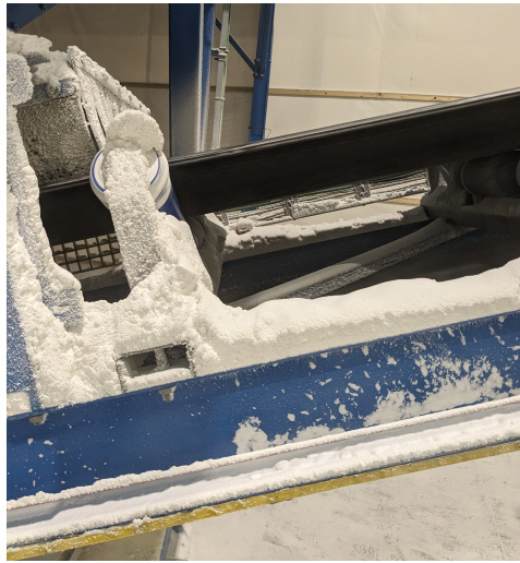
Figure 6.10: Dust settlement on equipment surrounding the reclaim bunker
