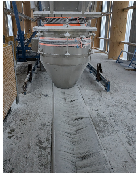
Figure 6.9: Dust settled on pathways and equipment surrounding the DSH used for warehouse loading
