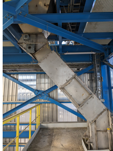
Figure 6.7: Transfer chute between conveyor belts
