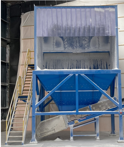
Figure 6.6: Reclaim with fabric dust collectors and dust curtain. Source: Verbrugge (2024)
