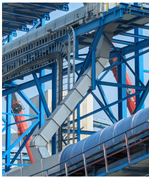
Figure 9: Transfer chute between two conveyor belts
