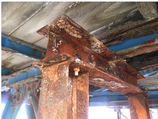
Figure 3.9: Corrosion at an old installation at Verbrugge
