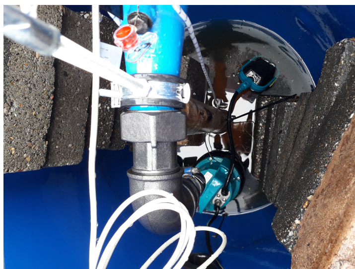
Figure D.1: Temporal single drain-water tank barrel 2. In this barrel the cable tie is not fixated to the pump itself but to the installed wooden pole in the barrel. This was required to activate the pump before the maximum water level inside the barrel was above the water level in the ditch.
