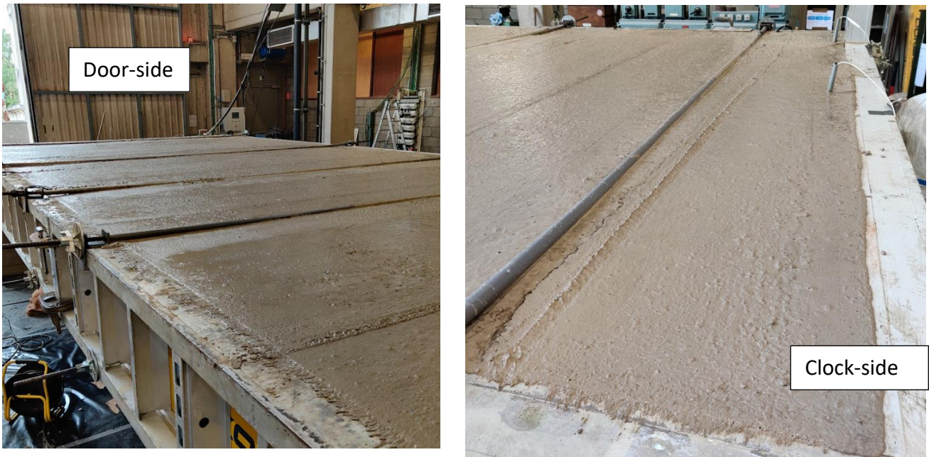
Figure 3-11: Pictures taken after the topping of the mock-deck has been cast, showing the two named sides of the slab
