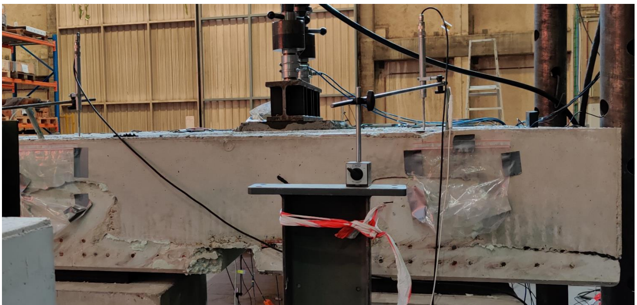
Figure 3-29: Photo taken from side D (clock side) of the test setup on 08/12/2021. Visible on the right: White fiber optic cable belonging to rebar Long 1
