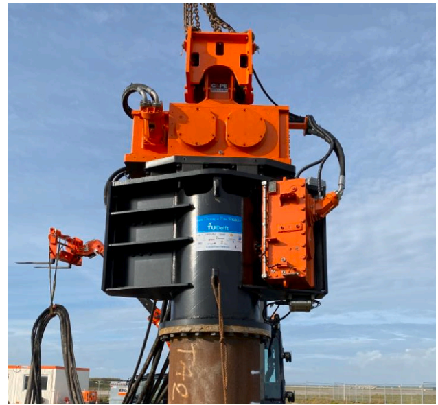
Fig. 1. The medium-scale GDP shaker connected to a pile via a bolted flange connection.
