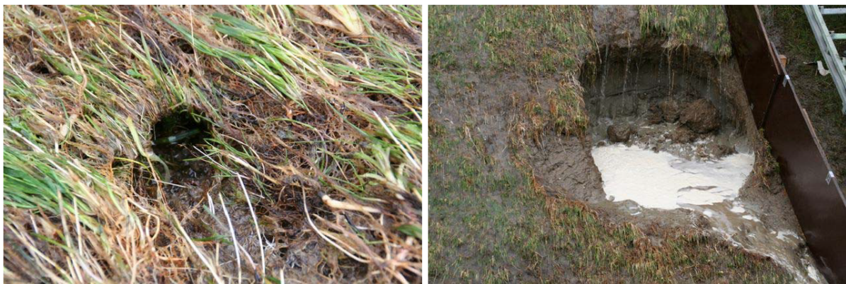
Figure A.6: Sint Philipsland. Slope failure after a simulation with a maximum load of 50 l/s/m overtopping waves (right picture). Failure from the slope of the dike, expected weak spot of a large mole hole remained intact (left picture).
