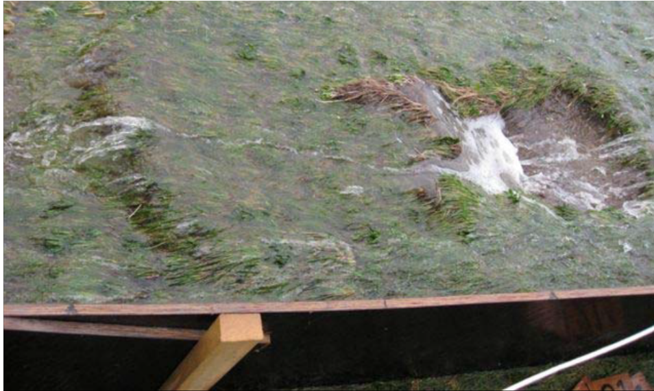
Figure A.2: Boonweg, section 3, initial damage. Slope failure of a saturated grass cover during a simulation, during the second hour of 75 l/s/m overtopping waves. The forcing of the water caused roots to snap, which enabled the formation of a protruding bulge filled with water under the grass cover. During further load the balloon burst and the grass cover flushed away.
