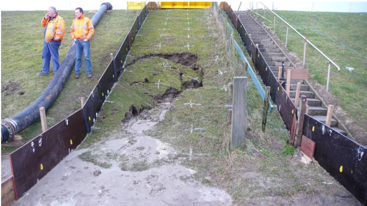
Figure A.8: Tholen, section 3. Failed slope after a simulation with a maximum load of 5 l/s/m overtopping waves. Failure shows macro instability: a large chunk of soil has slipped off. It is remarkable that a location at the slope cover was a weaker spot than the objects on the slope.
