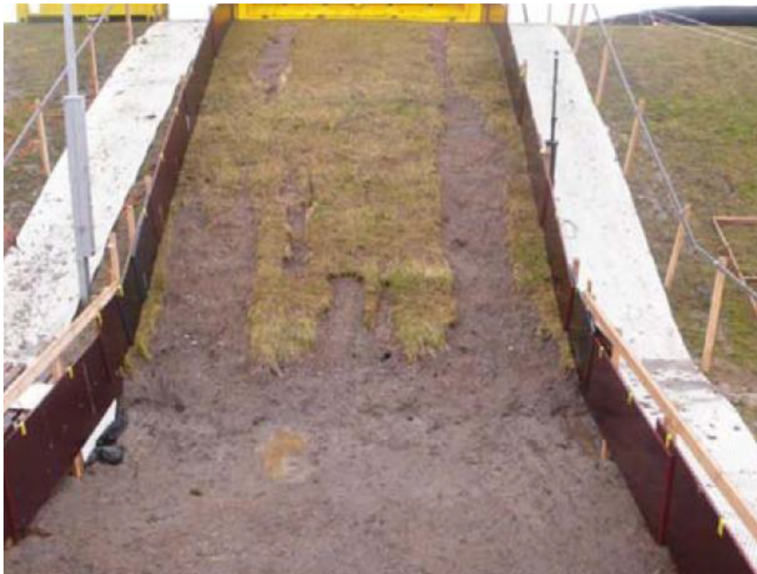
Figure A.1: Afsluitdijk, section 1. Final slope failure after 6 hours simulation with a maximum load of 75 l/s/m overtopping waves. Damage appears as rather even removal of the upper layer, starting at the toe of the dike and developing slope upward, but no hole develops.
