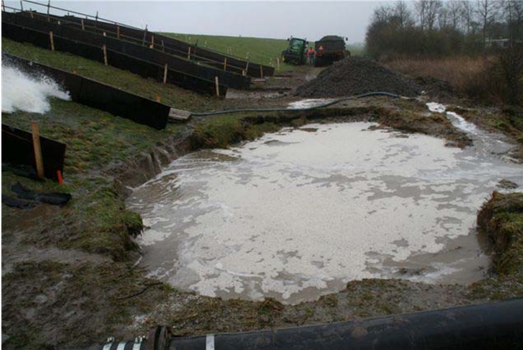
Figure A.5: Kattendijke, section 1. Slope failure after 5 hours and 40 minutes simulation with a maximum load of 75 l/s/m overtopping waves. Failure of the maintenance road down the toe of the dike, starting at the side away from the dike and developing towards the dike.
