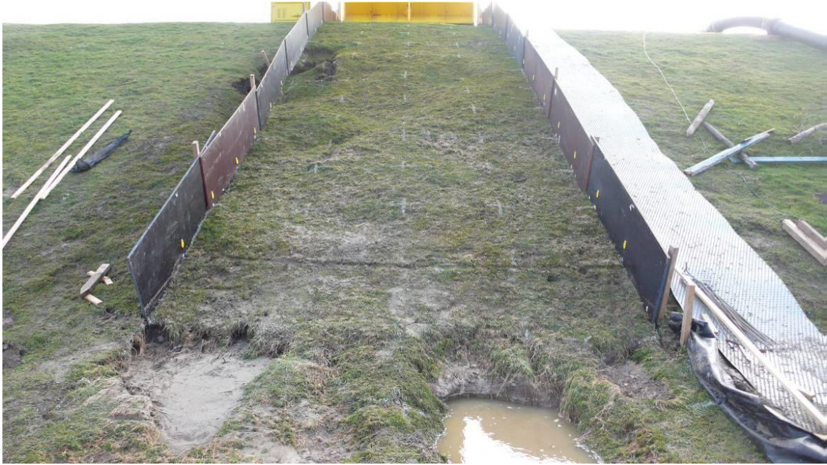
Figure A.9: Tholen, section 4. Slope failure after a simulation with a maximum load of 30 l/s/m overtopping waves. Failure at the toe of the dike, in the transition from the sloping to flat soil surface.
