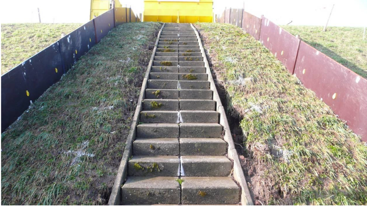
Figure A.7: Tholen, section 2. Slope failure during a simulation, after 1 hour of 5 l/s/m overtopping waves. Clear development of damage in the juncture between the soil cover and the stairs.
