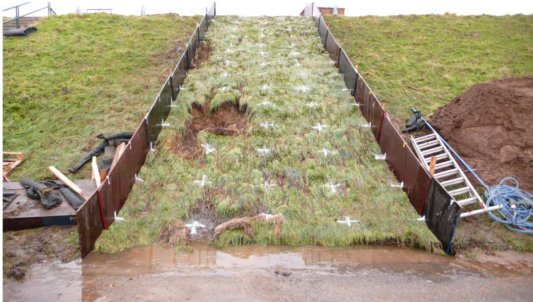
Figure A.11: Tielrode, section 4 . Slope failure after 3 hours simulation with a maximum load of 10 l/s/m overtopping waves. Start of failure of the slope cover at multiple locations.
