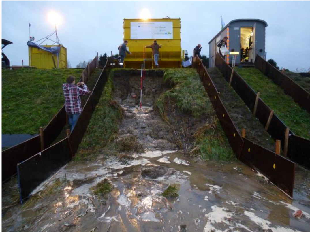
Figure A.14: Wijmeers II, section III. Slope failure after 1,5 hours simulation with a maximum load of 25 l/s/m overtopping waves. Failure started as a shallow damage (removal of grass cover over the total length of the slope) and eroded to the core of the dike.
