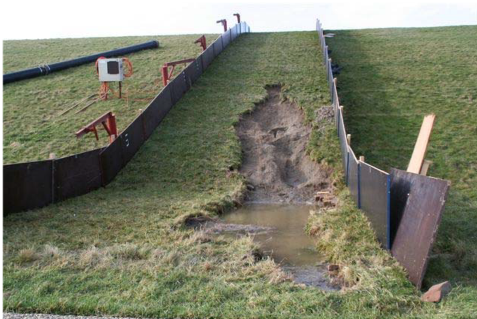
Figure A.3: Boonweg, section 3, final damage. Failed slope after a simulation with a maximum load of 75 l/s/m overtopping waves. Failure started halfway the slope of the dike and developed down the slope.
