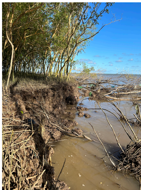
(b) Cliff erosion at the sea side of the mangrove forest.
