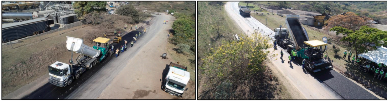
Fig. 8. Paving project having asphalt mixture containing recycled waste plastic in KZN province of South Africa [164].
