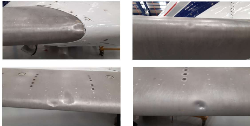
Figure 8: Sample of training data corresponding to dents of aircraft in Abu Dhabi Polytechnic Hangar
