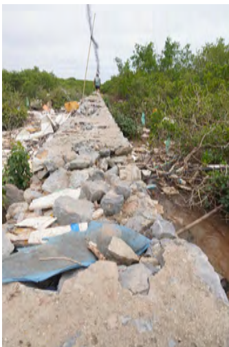
Figure 2.8: Holes in the Northern breakwater at Ngoc Hai.
