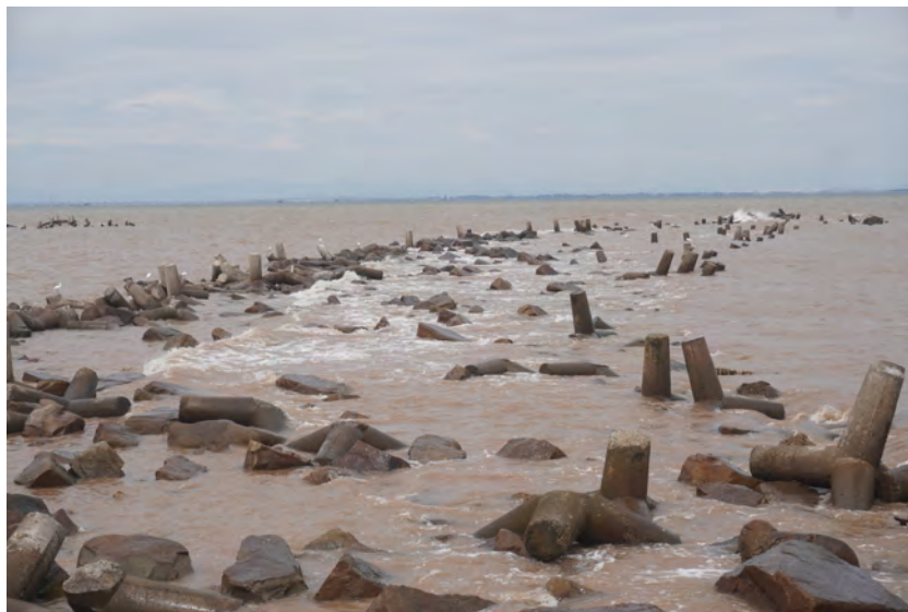
Figure 2.5: Southern breakwater at Ngoc Hai under wave loading from East direction (moving right to left) and high tide, overtopping does occur.
