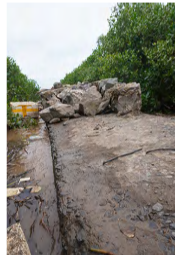
Figure 2.10: Shearing of 2 rock layers, Northern breakwater at Ngoc Hai.
