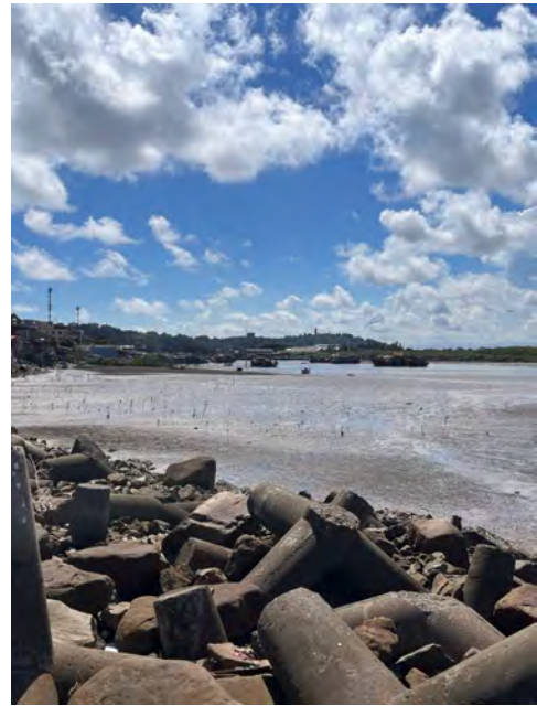
Figure 2.7: Broken tetrapods of the Southern breakwater.
