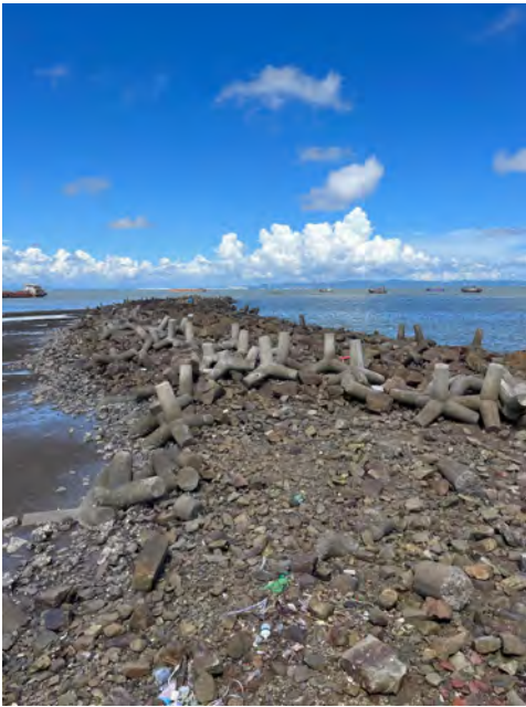
Figure 2.6: Stone sizes and tetrapods of the Southern breakwater.
