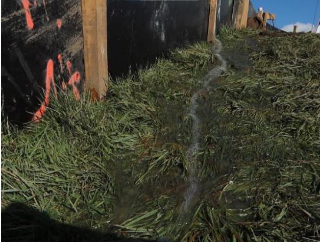
Figure 29 Water flowing under wooden side boards
