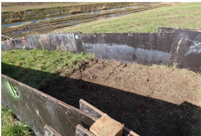
Figure 9 Upper damage dike (removal of 2x2m grass layer)
