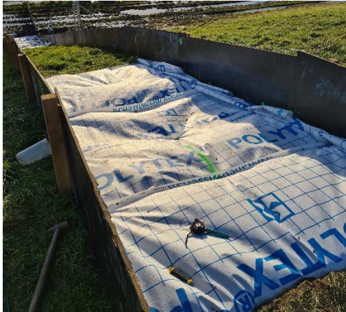
Figure 2 Installed plastic sheets on upper damage (plastic sheet in figure is Polytex®, not Tyvek®)
