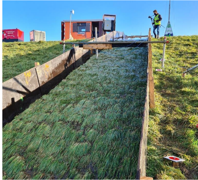
Figure 30 Grass between two damages after overflow test were performed
