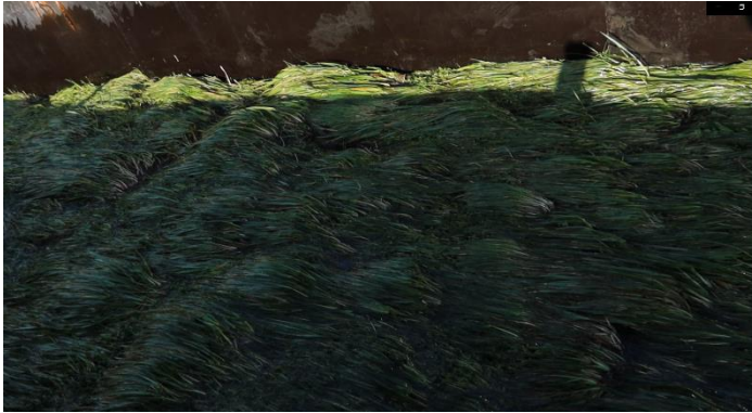
Figure 23 Grass between two damages after overflow tests
