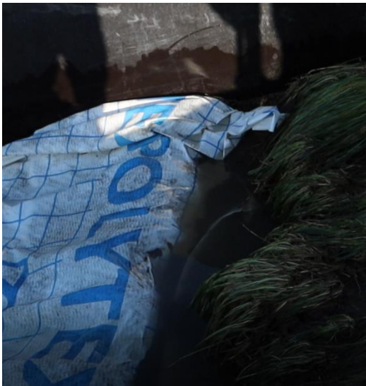
Figure 24 Trench at lower damage after overflow tests
