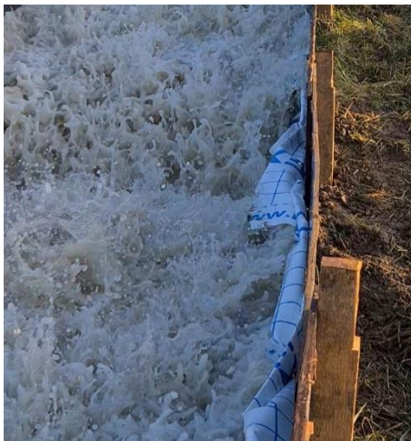
Figure 31 Water-overflow at the boundary with the wooden panels
