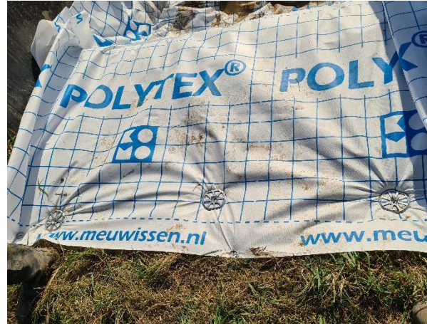
Figure 3 Installed sheet with anchors lower damage (plastic sheet in figure is Polytex®, not Tyvek®)
