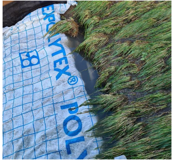
Figure 33 Trench at lower damage after overflow tests were performed
