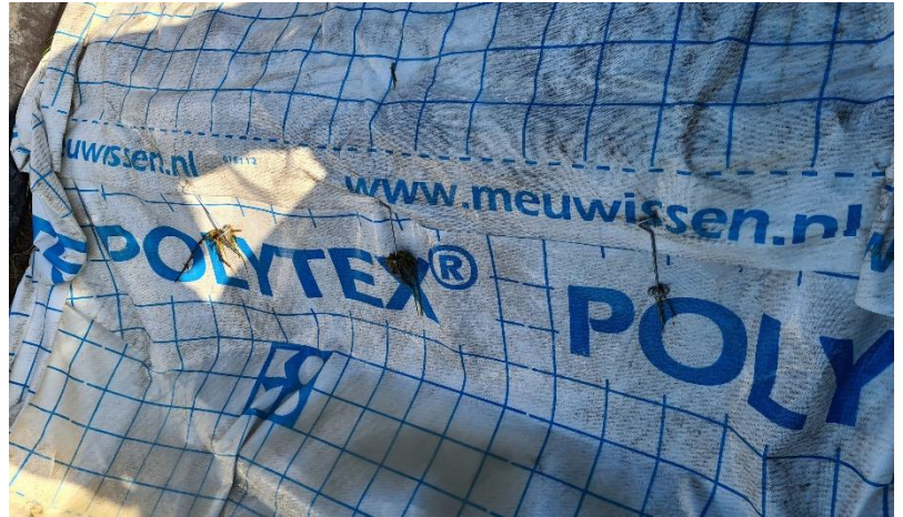
Figure 28 Lower damage after overflow tests were performed
