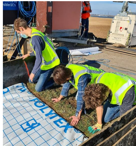
Figure 4 Flipping back of grass layer over the sheet at the upper damage (plastic sheet in figure is Polytex®, not Tyvek®)
