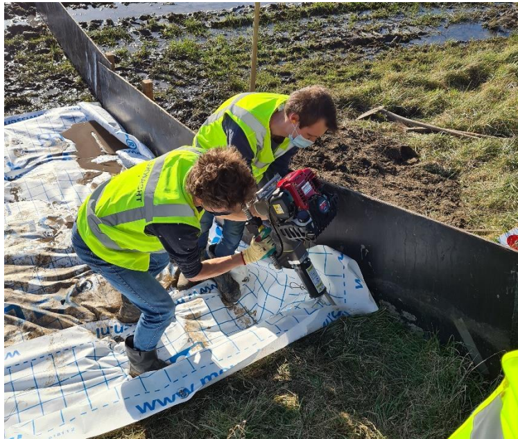
Figure 5 Drilling of TL-DTOOL anchor installation rod with GPD at upper damage (plastic sheet in figure is Polytex®, not Tyvek®)
