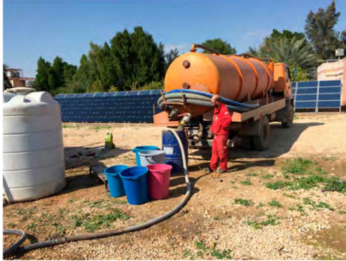
Figure 42: Septic tank sludge conveyance (photo taken by H.A. Garcia Hernandez)
