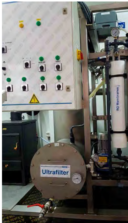
Figure 41: Ultrafiltration and reverse osmosis unit
