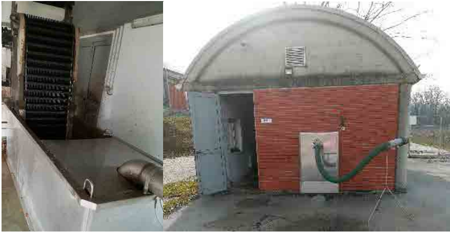
Figure 24: Septic tank sludge intake station at WWTP (Ptuj, Slovenia)
