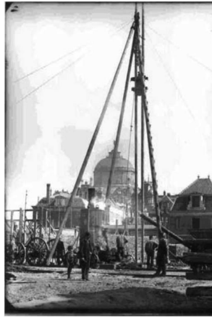
(b) Usage of the steam engine for pile driving. Photo taken by Jacob Olie, 1891, Reprinted from Korff, M. (2012). Response of piled buildings to the construction of deep excavations (Doctoral dissertation). University of Cambridge. IOS Press BV
