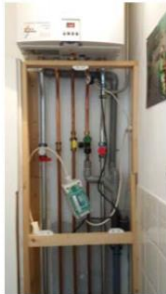
Figure 4.2: Eltako Electricity meter used for measuring in real time the combi-boiler's pump energy consumption. (Source: Monicair report)
