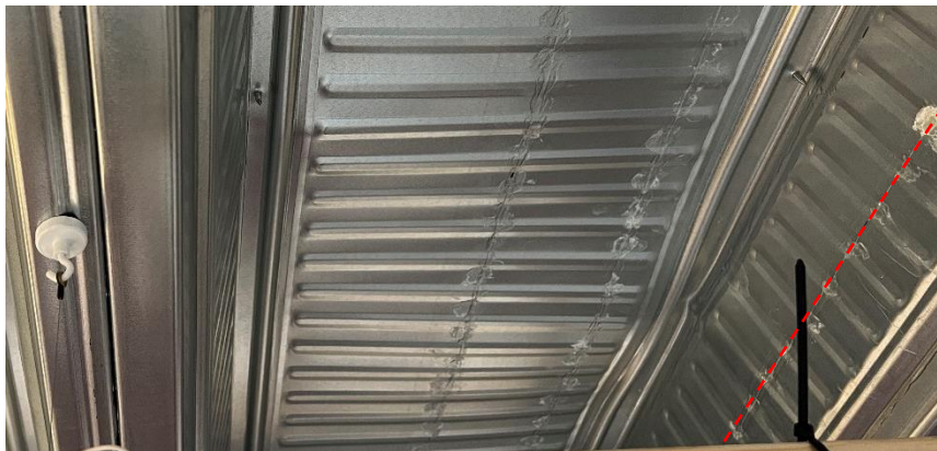
Figure 6.9. Buckling of the steel sheeting of Slab 11.
