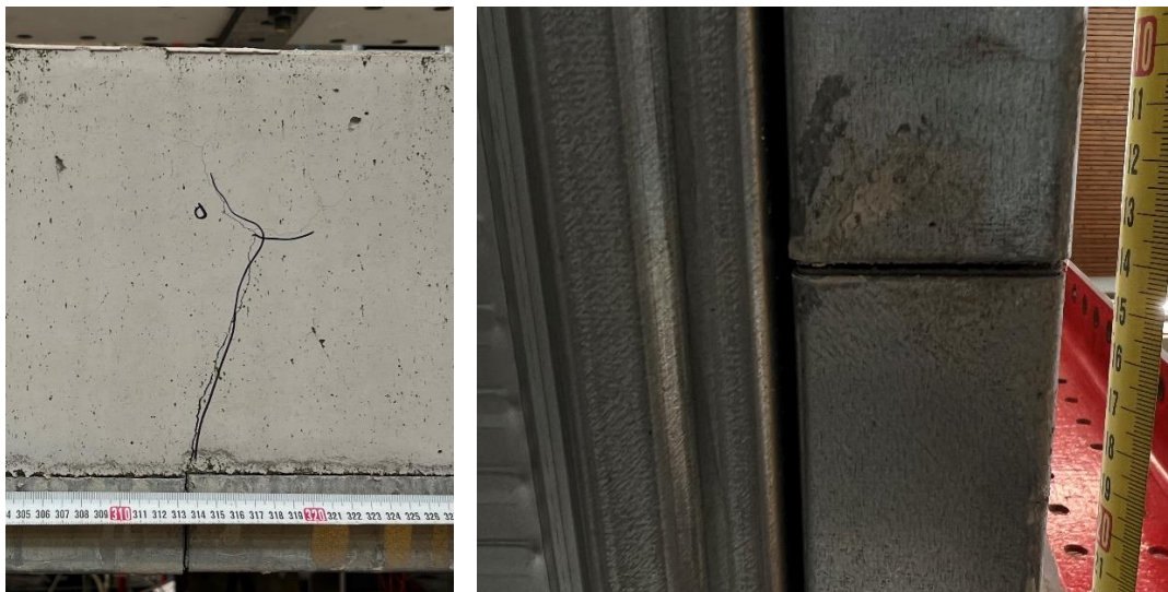
Figure 7.4. Side view (left), and bottom view (right), of the gap in the steel sheeting.
