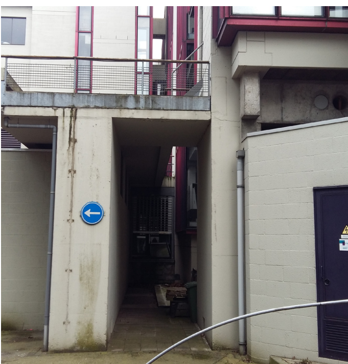
Fig. 157: On the right the added technical room under the island and on the left the other added technical room.
