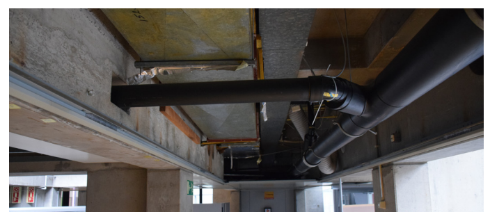
Fig. 37: Rainwater pipe going through an extra hole in the beam.
