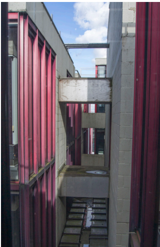
Fig. 147: Space between technical tower en facade, covered pipes.
