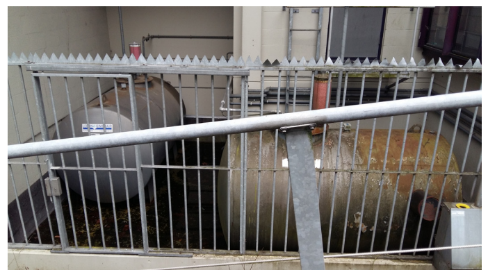
Fig. 158: Oiltanks likely used as backup generators.
