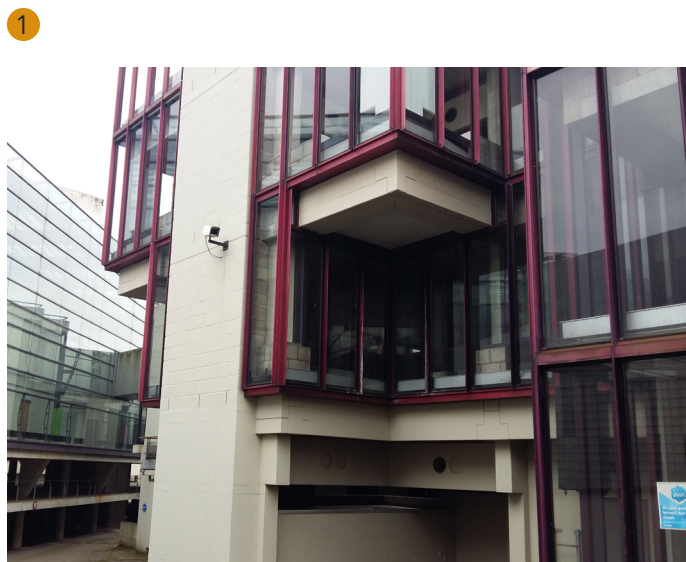
Fig. 221: Disorder in the facade on the first layer.
