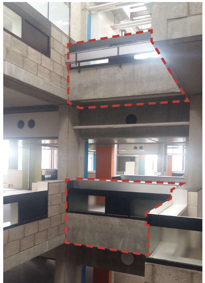
Fig. 197: Photograph of two examples of the bridge extensions above each other (dashed red).
