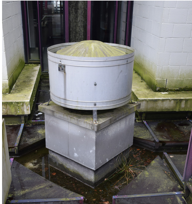
Fig. 74: Ventilation unit at a cross section of two gutters.
