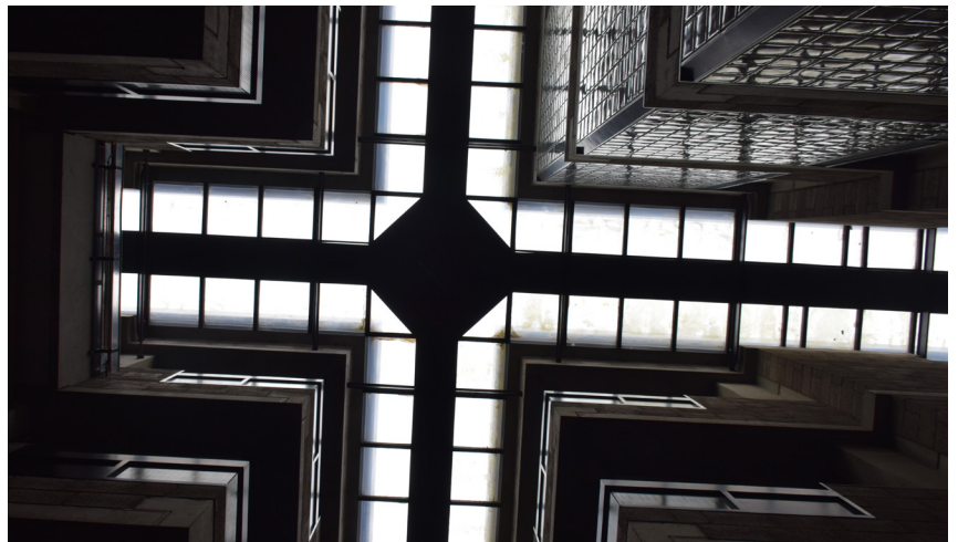
Fig. 73: Picture of the gutter and skylight as seen from inside the building.
