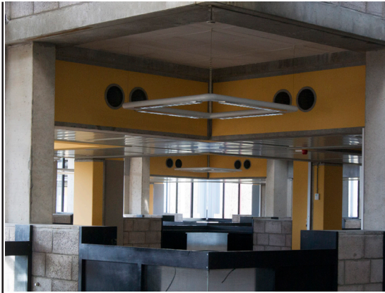
Fig. 31: Frengerceiling in a workplace.
