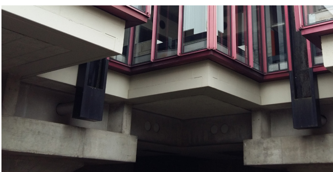
Fig. 38: Rainwater drainage on the facade going back in the building.
