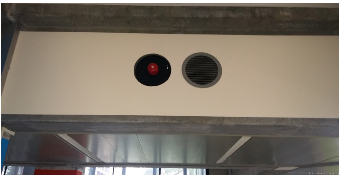
Fig. 35: A ventilation grille and a fire alarm on the spot of the openings.
