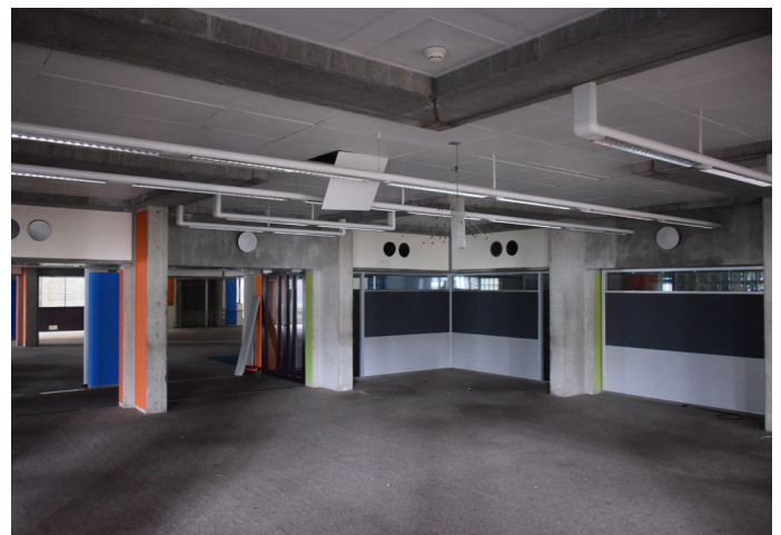
Fig. 218: Inner walls in computerroom.
