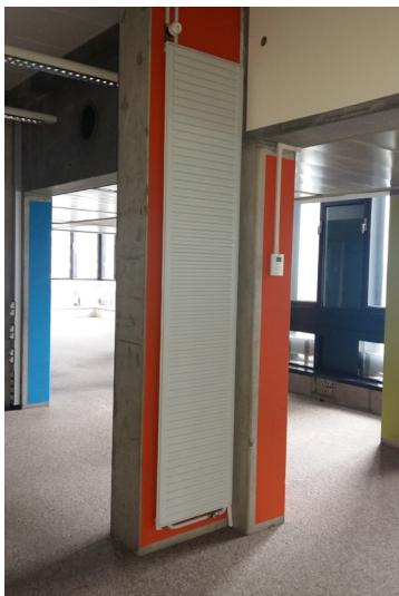
Fig. 215: Radiator in computerroom.
