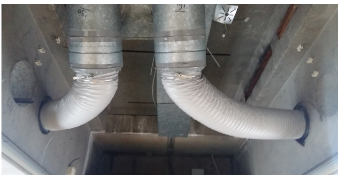
Fig. 36: Ventilation tubes between the primary beams.
