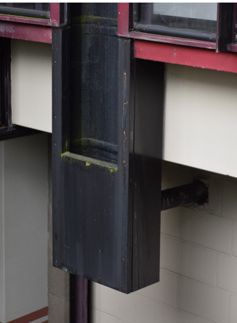
Fig. 75: The end of the gutter and the continuation of the rainwater drainage.
