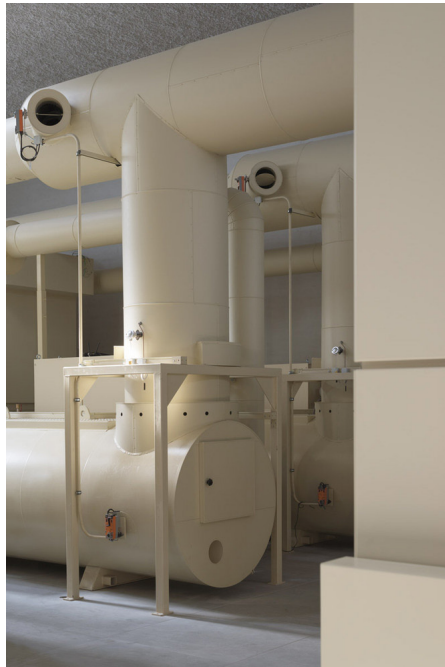
Fig. 44 - Technical installations are made visible for the visitors to give them the opportunity to be part of the final moments of their loved ones. The installations are coloured in yellow to give a more calm atmosphere (Bossi, 2018)
