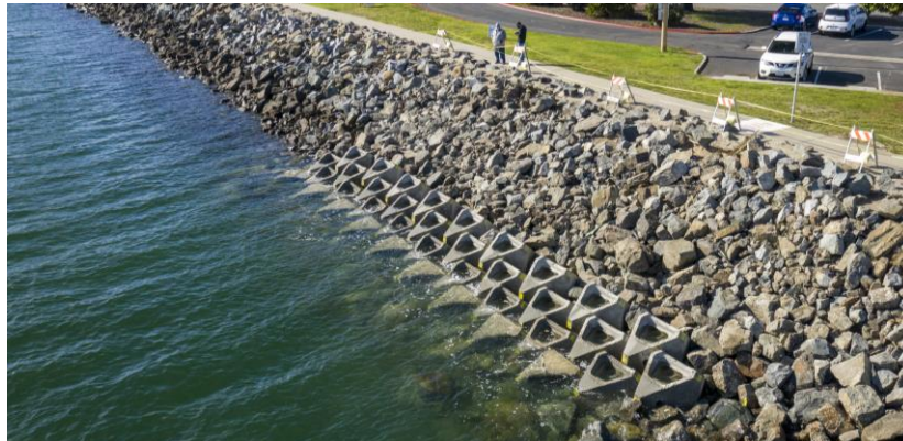
Figure 2. Inaugural deployment of Coastallock unit at the Port of San Diego (PoSD)
