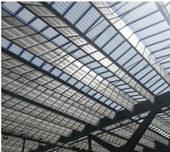
Integrated solar panels
