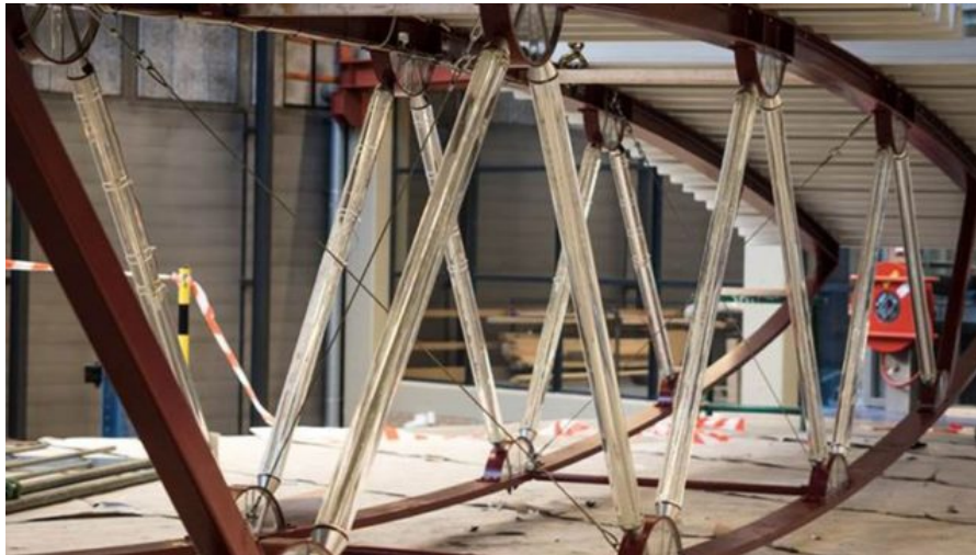
Figure 1.2: Picture of the Glass Truss Bridge designed by researchers of Delft University of Technology before erection. The diagonals consist of bundled glass rods [3].
