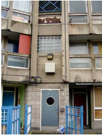
Figure 25. The exterior façade showed the corrosion in the concrete reinforcement. (Peter Stewart Consultancy, "Robin Hood Gardens," 9.)
