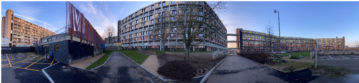
Figure 28. Current state of Park Hill in December 2021 with externally unaltered blocks on the left, blocks under renovation in the middle, and renovated blocks on the right. (Photograph by Author).
