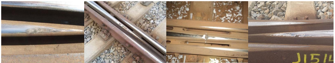
Figure 3 - Examples of damaged crossings [1] [2]
