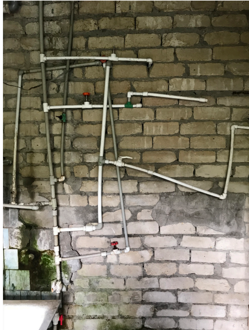
Figure 13_ Plumbing in a Shared Bathroom in the Main Block
