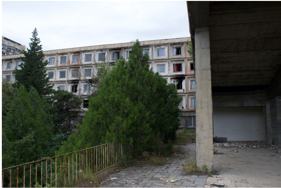
Figure 11_ Charred Facade of Main Block
