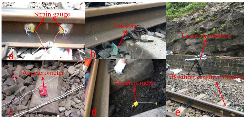
11 Fig. 6 Detail of track instrumentation at transition zone: (a) dynamic load on rail; (b) rail seat loads; (c) sleeper acceleration; (d) 12 special box for accelerometer in ballast bed; (e) sleeper displacement 13
