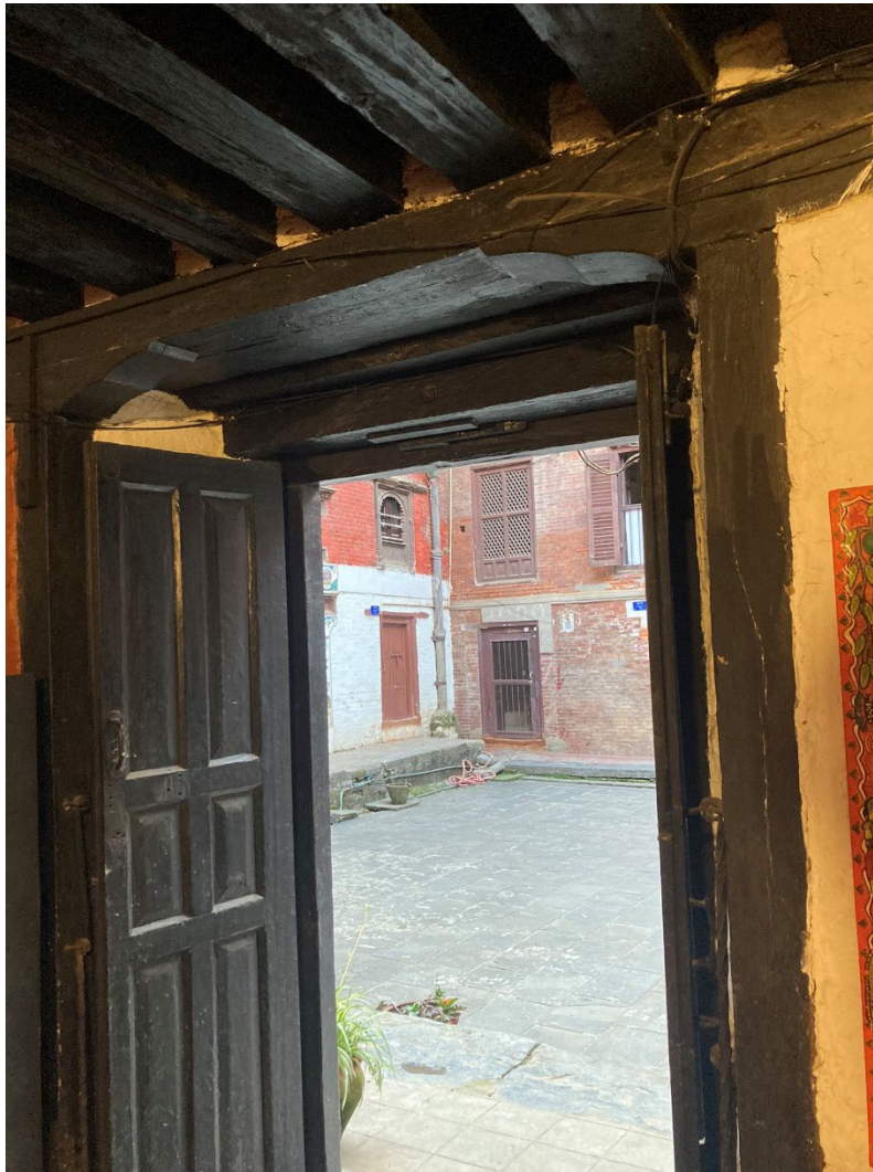
Figure 12: Details of the interior of the Malla-era Newar house: Hira Guesthouse. Vertical timber posts in corners, strong window frames, horizontal timber beams embedded in the masonry, thick walls, wooden floors and low ceiling heights. It is no wonder this building has survived three major earthquakes already. (Author's own photograph, 2023).
