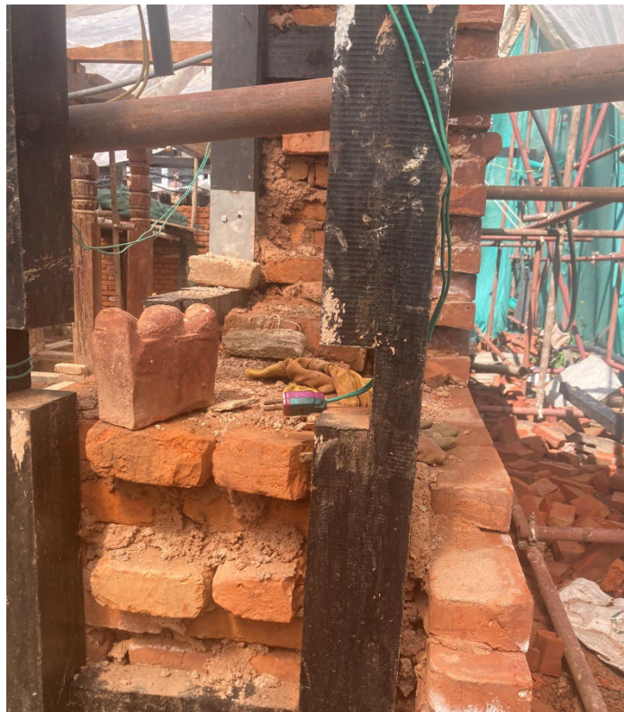
Figure 13: Construction of a wall of the Ikhachhe Bahi temple in Patan, as a part of the reconstruction of the temple. The wall thickness is achieved by multiple layers of brick, of which the outer layers exist of slightly tapered bricks (Author's own photograph, 2023).
