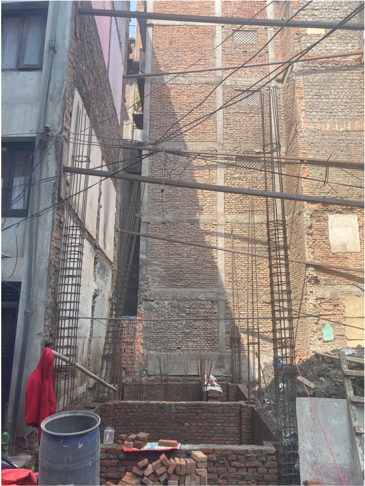
Figure 24: A category-3 (ERRRP, 2011) building is constructed in Patan. The columns and beams are of reinforced concrete, with brick infill-walls masoned in between. (Author's own photograph, 2023).
