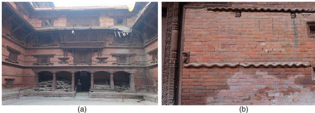
Figure 27: Visible timber ring beams and beams embedded in the masonry at the Hanuman Dhoka Palace in Kathmandu (Joshi and Kaushik, 2017).
