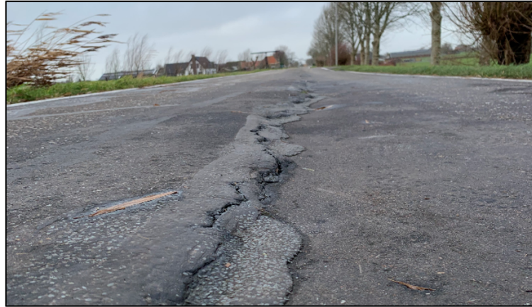
FIGURE 8.4: A picture made at the northern side of the Kwakelweg. The asphalt had cracked at numerous locations. The dimensions of the crack indicate that a problem concerning macro-stability of the dike is the cause.
