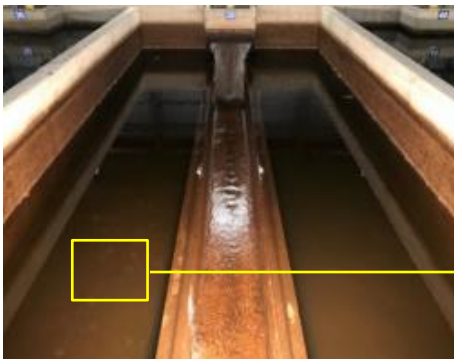
Figure 97a Full-scale RSF during ETSW 5 m/h up-flow
