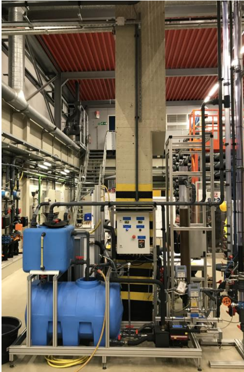
Figure 9 Waternet expansion column in Amsterdam
