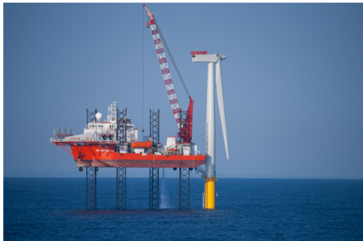
Figure 2.3: Installation or maintenance on a bottom-fixed wind turbine using a jack-up vessel
